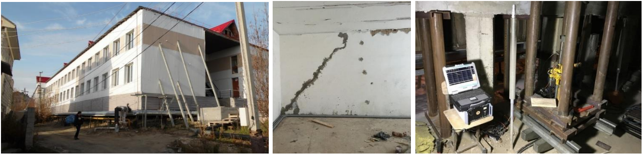
Figure 11. Salekhard College built in 1970s started experiencing deformations in 2014. 3 CPTs with total length of 12 m (including 10 m of frozen soil) and 8 temperature measurements were performed in the crawl space (1.9 m) under the structure. The initial hypothesis of thawing permafrost was not confirmed 19 .
