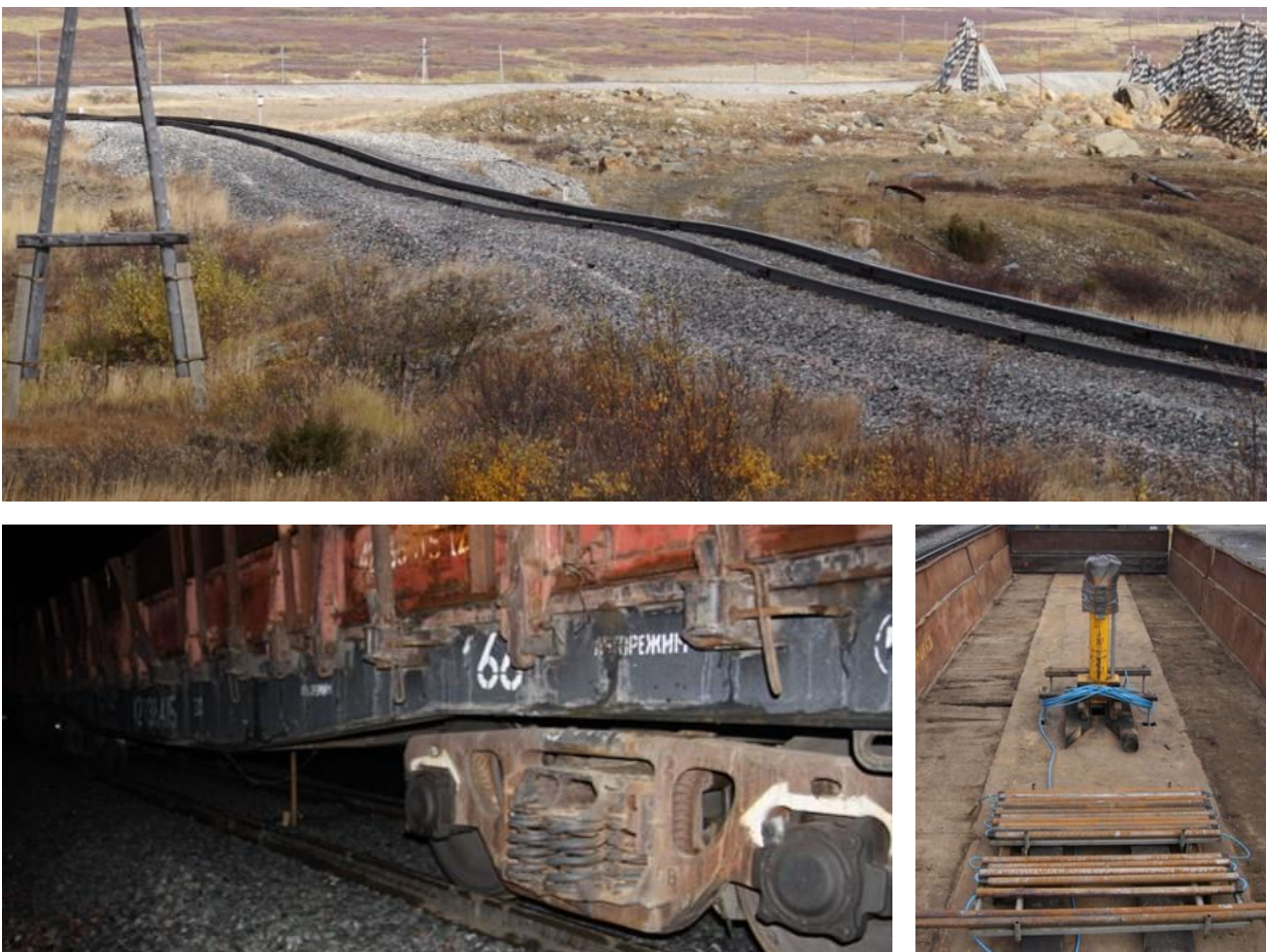
Figure 10. Differential settlement of the operational railway line near Vorkuta. 1 CPT with total length of 12 m (including 8 m of frozen soil) and 6 temperature measurements were performed at night within 3 hours. The initial hypothesis of thawing permafrost was not confirmed.
