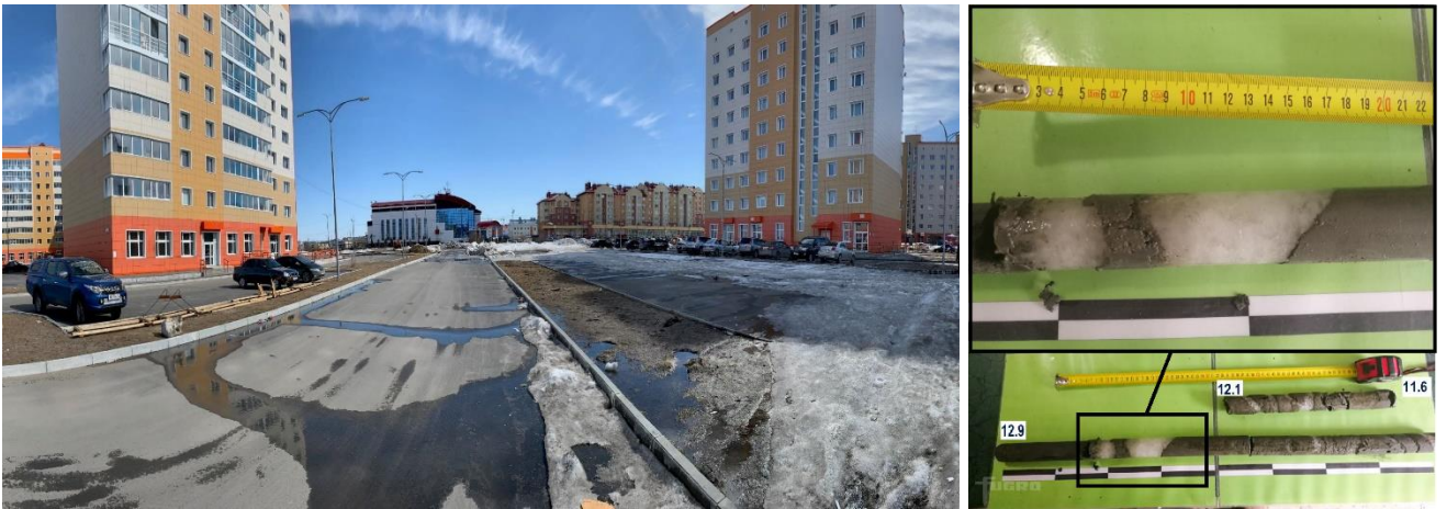
Figure 12. A multistorey apartment building in Western Siberia, erected in 2017, experienced differential settlement of up to 3 mm/month. 34 CPTs with total length of 724 m (including 360 m of frozen soil) and 305 temperature measurements were performed. Soil sampling showed ice lenses up to 10 cm thick, and the cause of settlement was found to be the thawing of the ice lenses.
